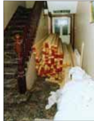
Figure 9: A blocked corridor with incorrect signage
